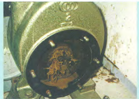
Clogging inside pump
